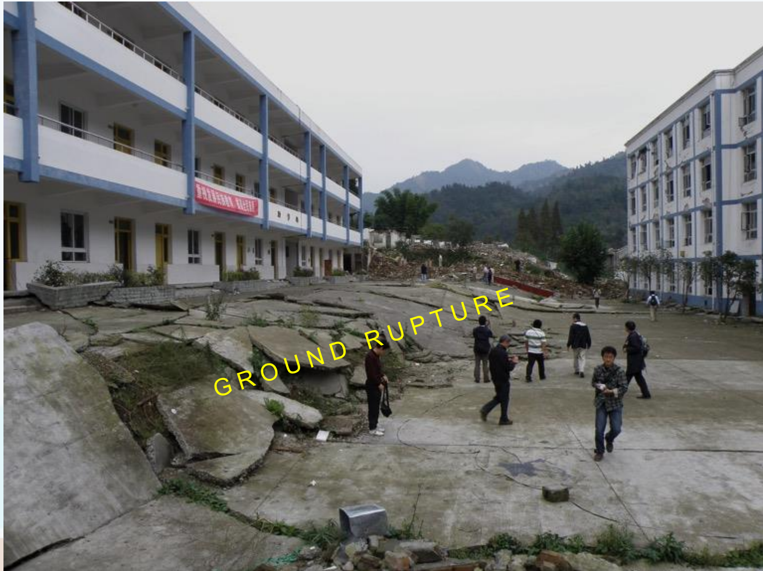
Bailu school, looking northeast in direction of rupture Photo credit to Dr. Gary Gibson
