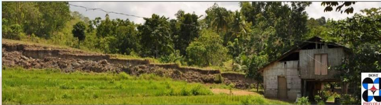
3-meter fault scarp of the North Bohol Fault in Brgy. Anonang, Inabanga
